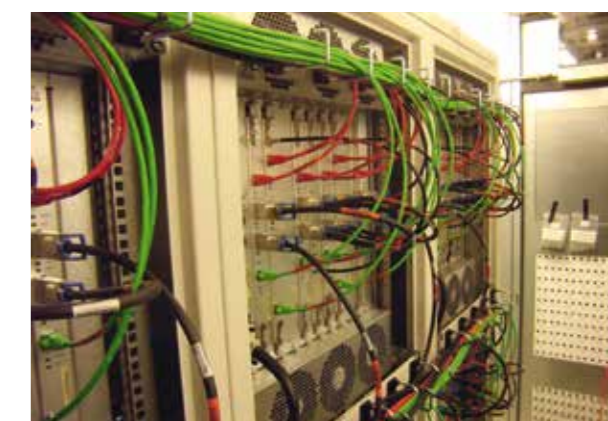
Fig. 1: Electronics in the station cabinet.
